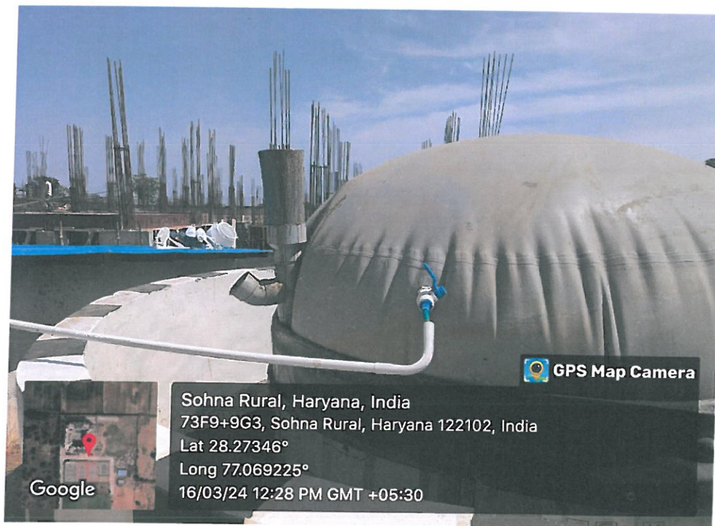
Figure: Inlet-side of Biogas plant
