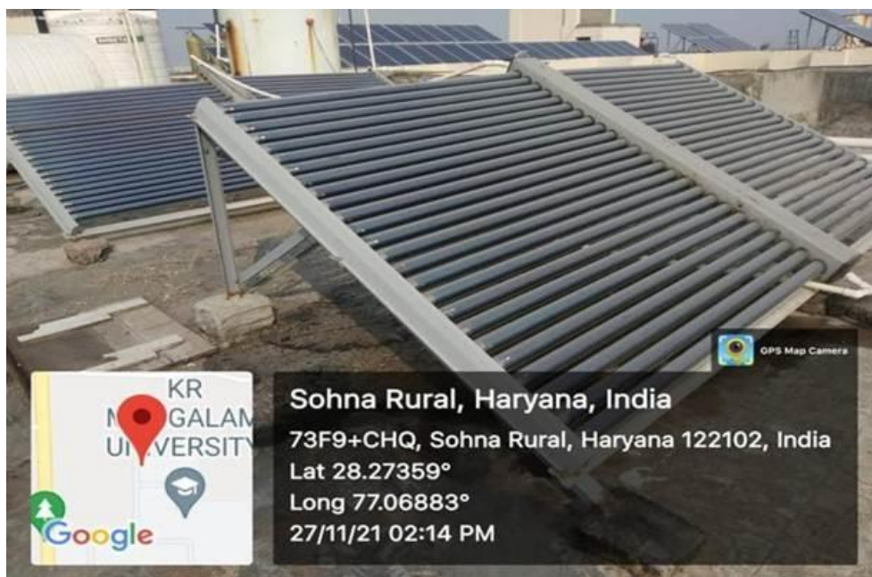
Solar thermal system providing hot water in hostels, reducing LPG and grid energy dependence
