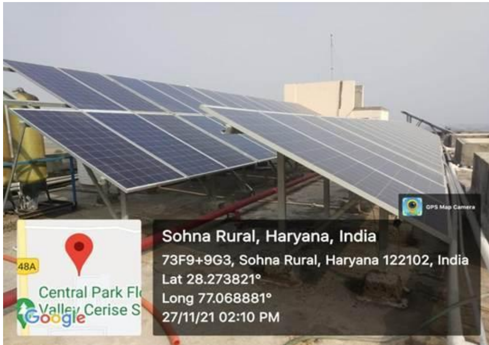
310 kWp rooftop solar PV system across Academic Blocks and hostels, generating clean electricity and reducing dependence on grid power
