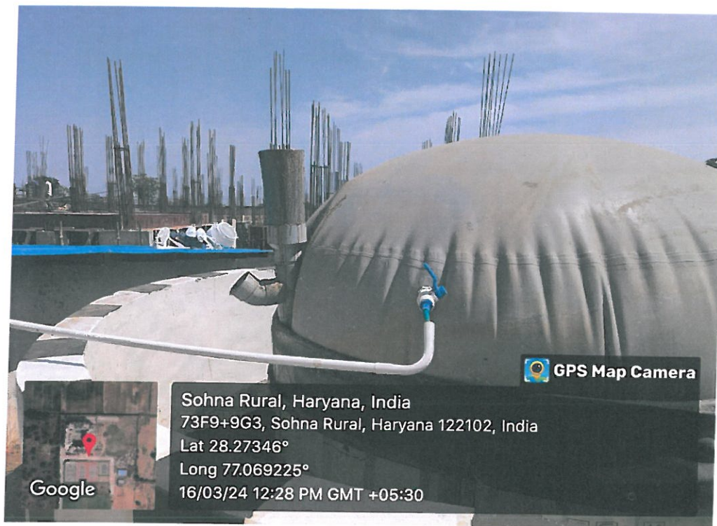
Figure: Inlet-side of Biogas plant
